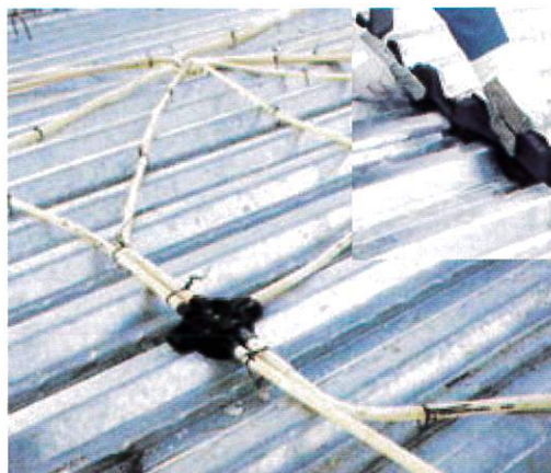
M&E accessories (i.e. pipe electricity appliances) to be installed upon laying of steel decking
